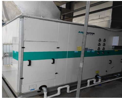
Upgraded constant temperature and humidity cabinets
