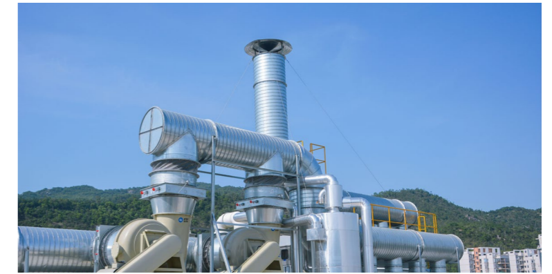
Waste gas absorption equipment inside the workshop and outside absorption tower of Multek Electronics
