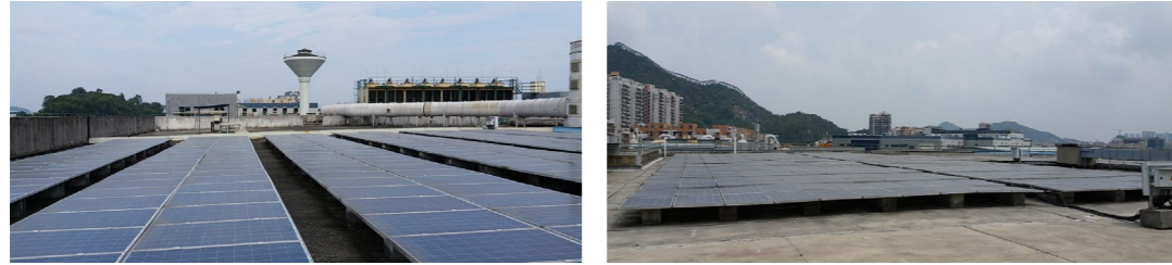
Solar panels on the roof of plants
