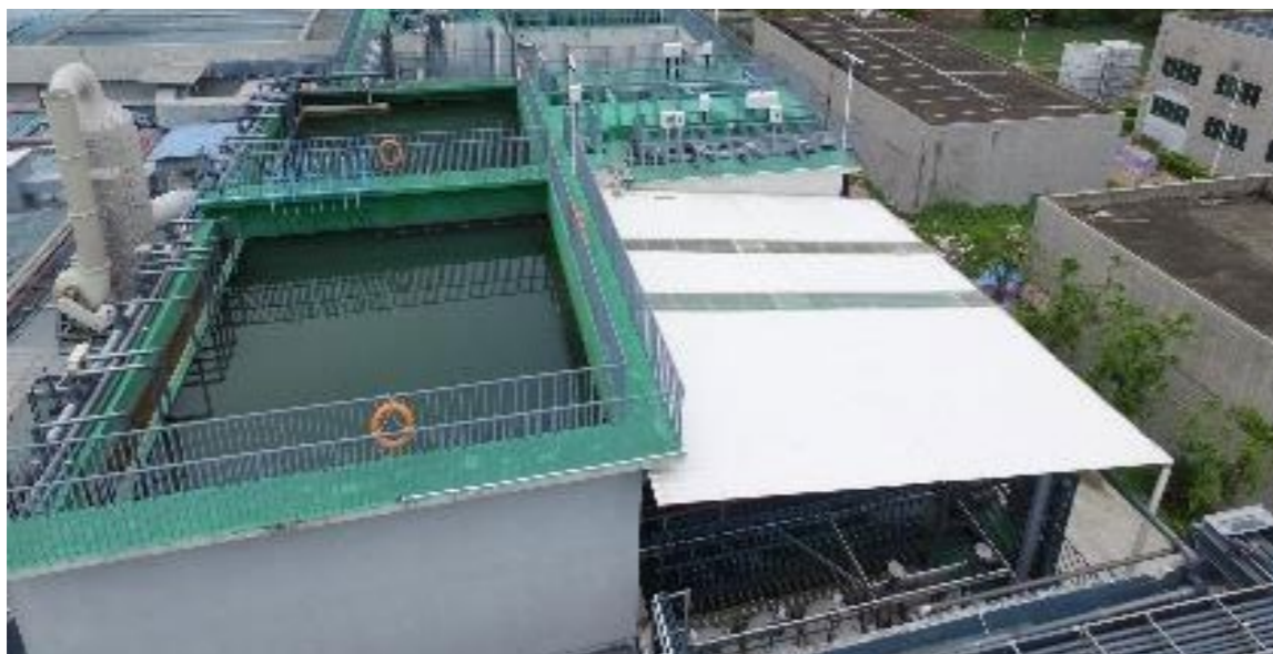
Wastewater treatment system
